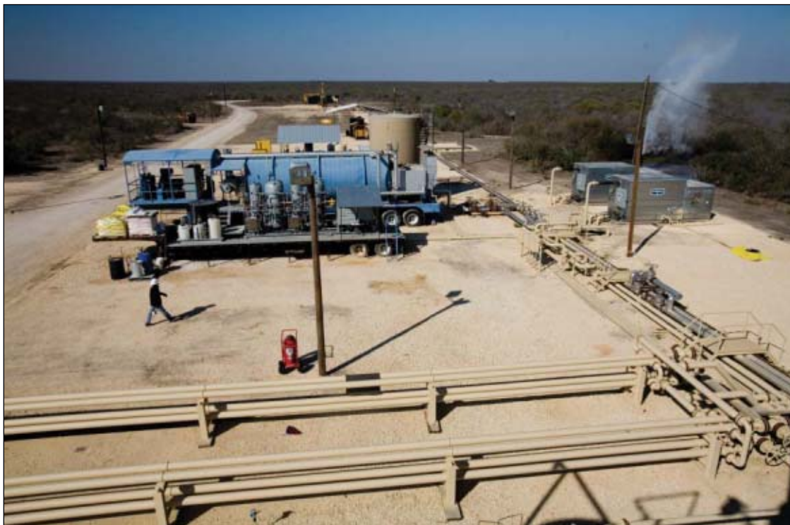
Gas-fired steam generator and tank battery at TXCO Resources-Pearl E&P two-well tar sand pilot in Maverick County, Tex. Photo courtesy of TXCO.
